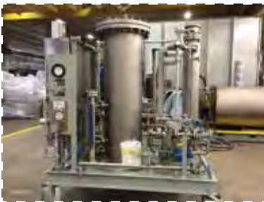
Ex: Stainless and Carbon Steel heated system with Pre-filter. Explosion-Proof with purged electrical enclosure and transmitters. 2014
